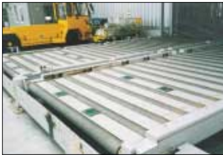
Lufthansa Cargo Center, conveying line
